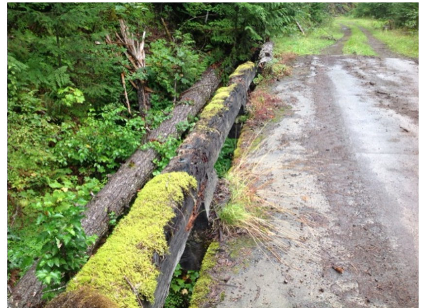
remaining guardrail condition
