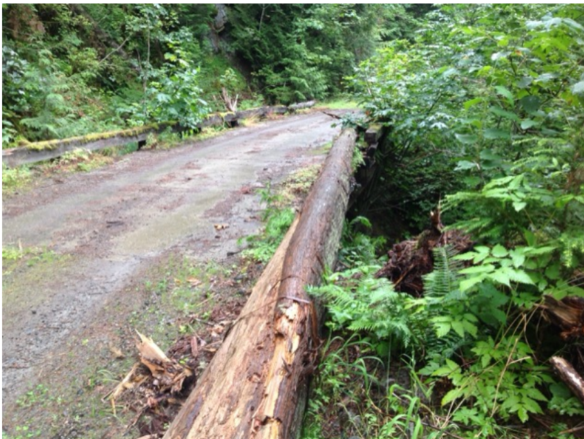
guardrail off and log has been placed
